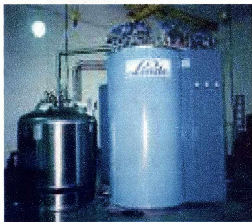
New Liquefier (200l/hr) installed at TIFR
