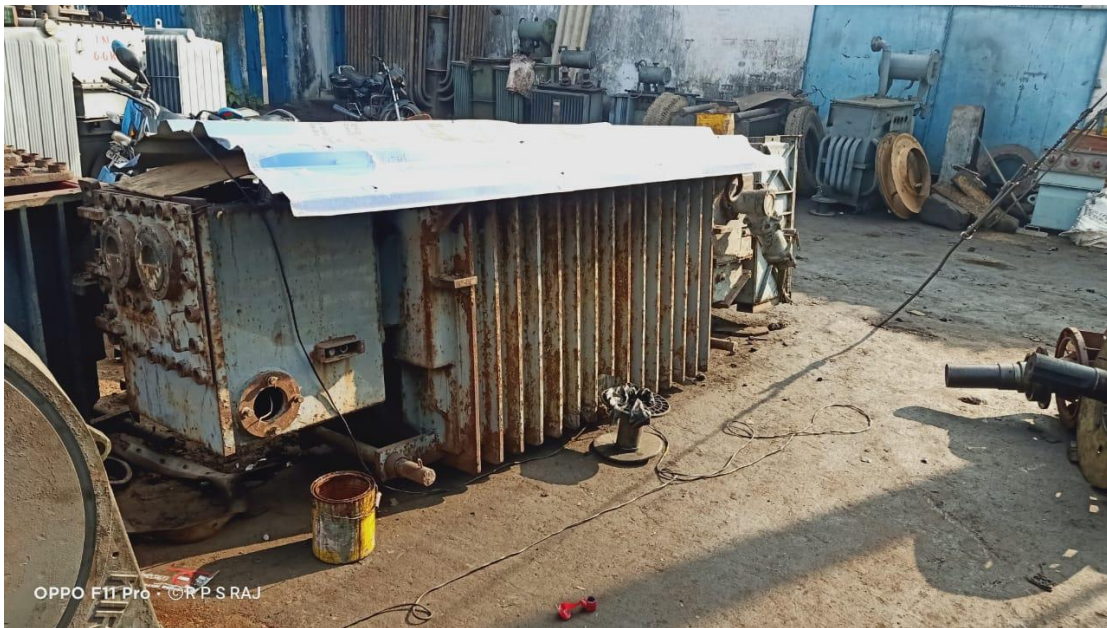
Fig. 4.14.: Used transformers for remanufacturing
